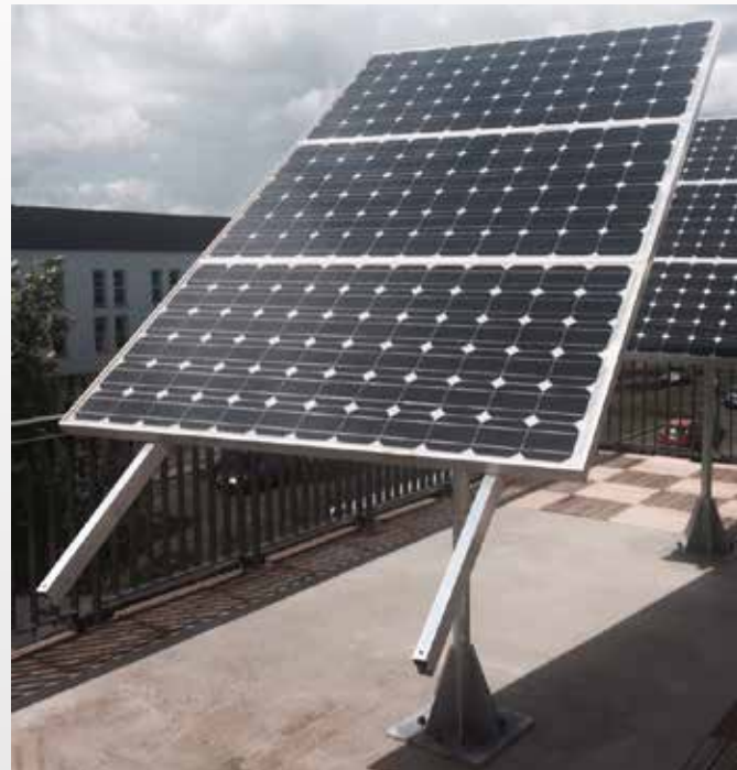
Solar tracker for 3 panels, 1,6 kWp. Quantity of trackers: 2
