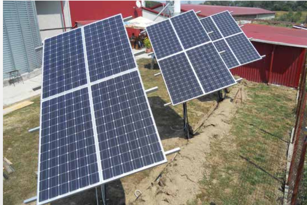
Solar tracker for 4 panels, 3,4 kWp. Quantity of trackers: 3.
