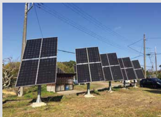
Power plant with an installed power of 6,6 kWp. Quantity of trackers: 5.
