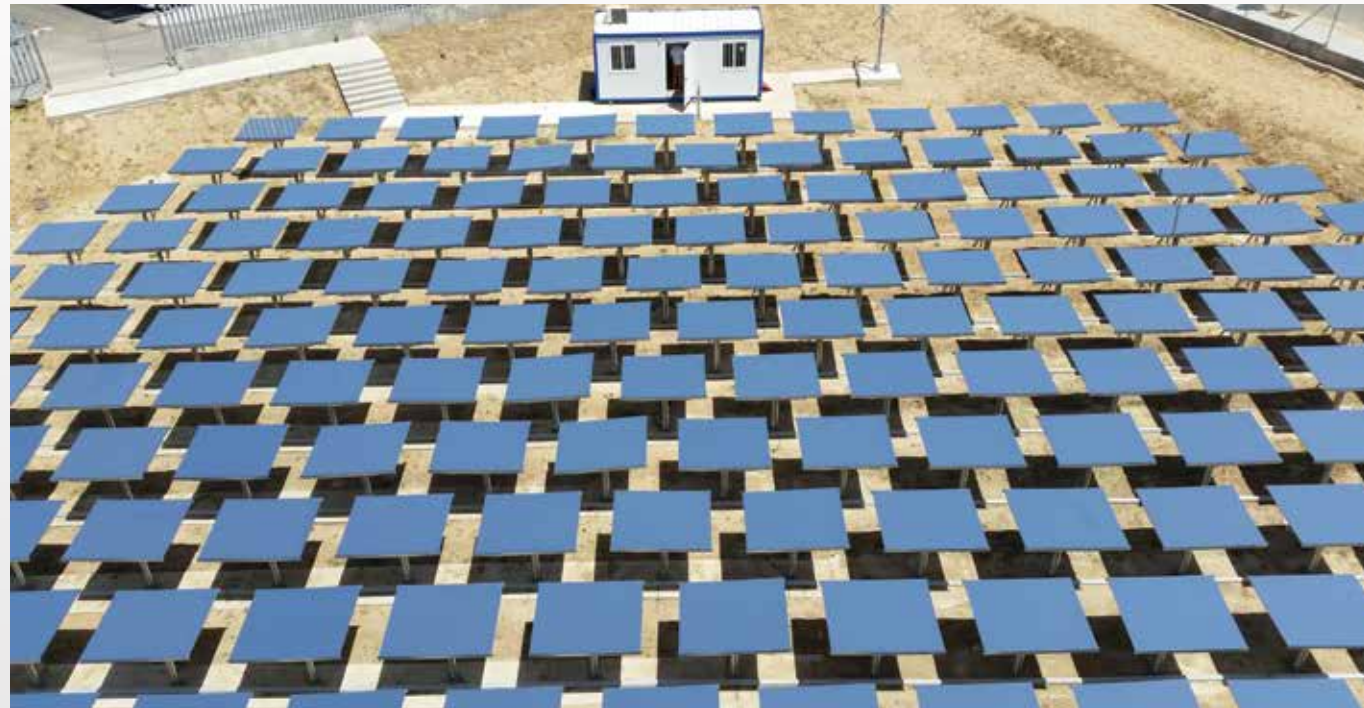
Heliostat field. Quantity of heliostats: 170.
