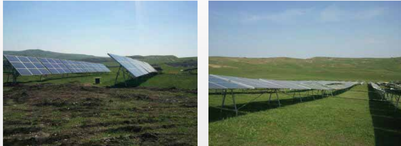
Power plant with an installed power of 3 Mega Watt.
