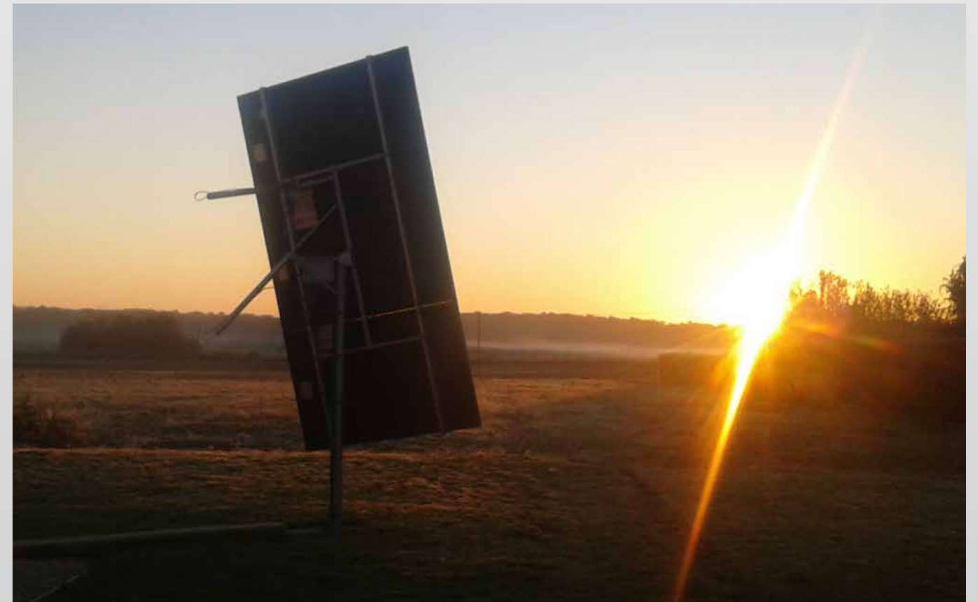
Solar tracker for 3 panels, 0,8 kWp.
