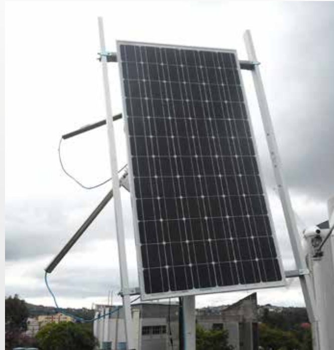
Solar tracker for 2 panels, 0,6 kWp.
