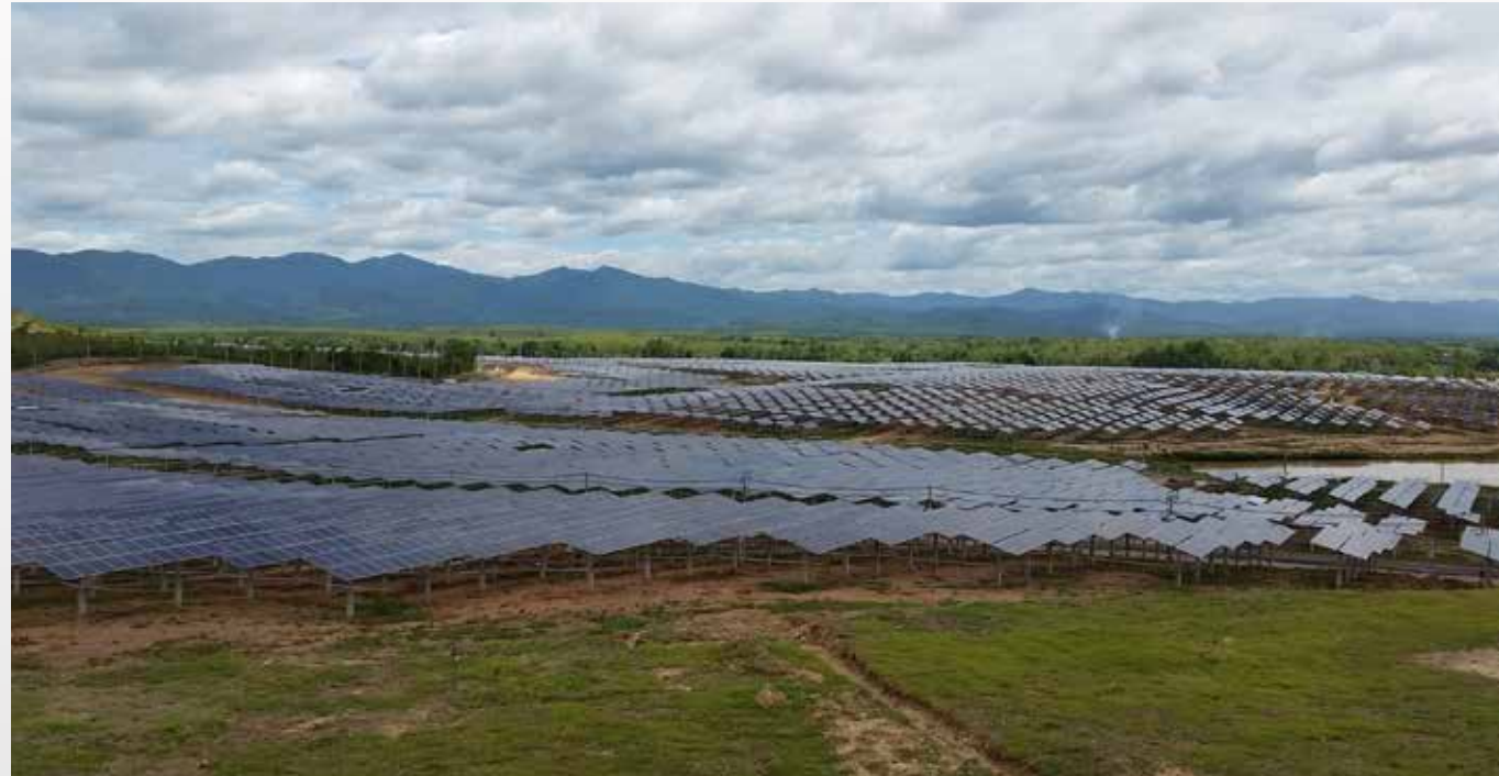
Power plant with an installed power of 120 MW DC.
