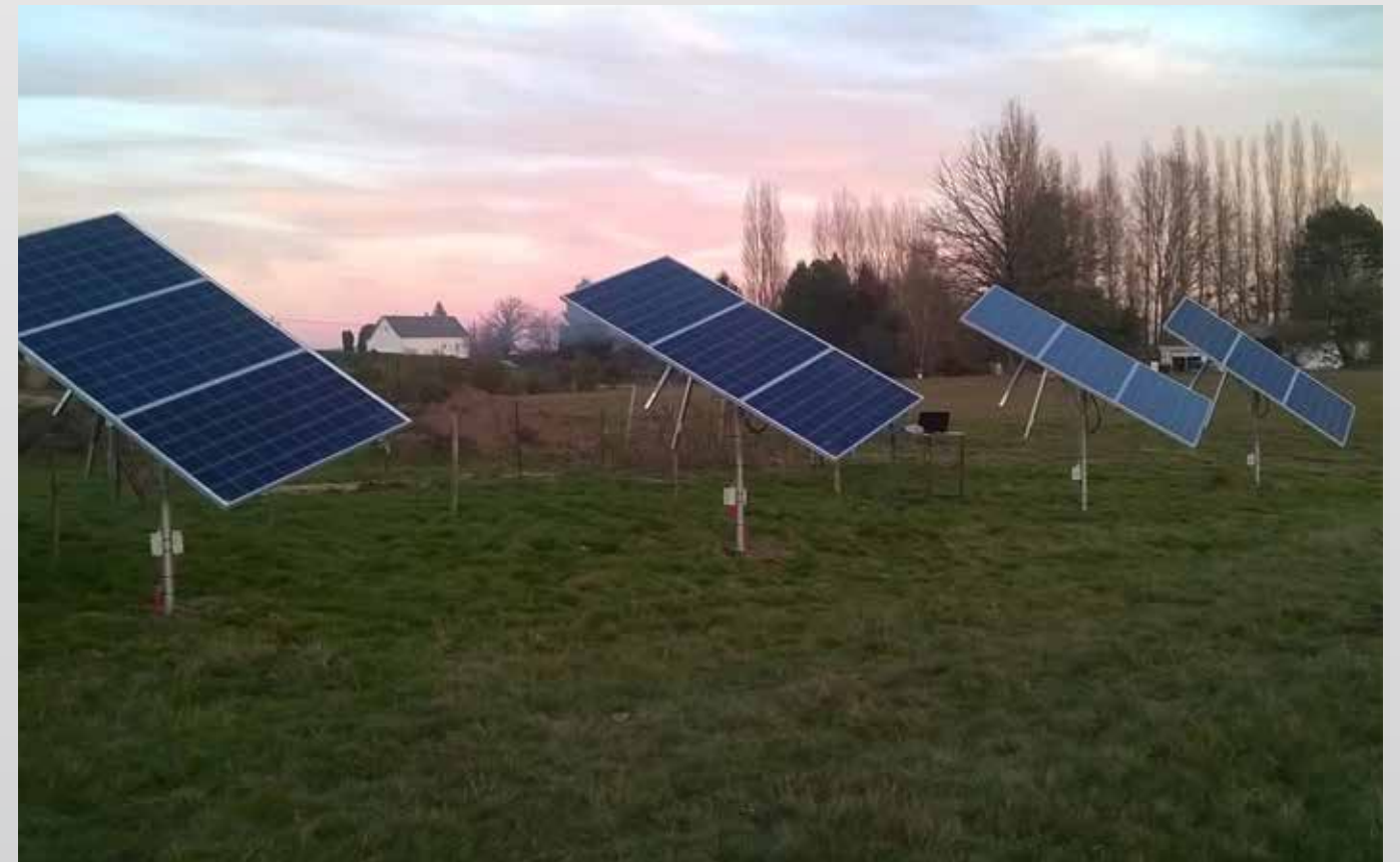
Solar tracker for 3 panels, 3,3 k Wp. Quantity of trackers: 4
