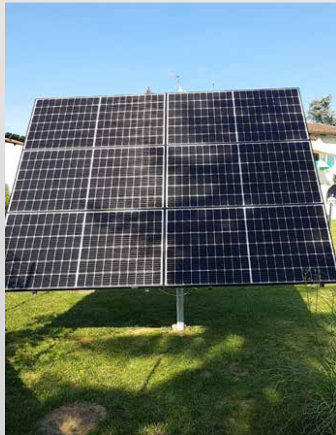
Solar tracker for 12 panels, 3,3 kWp.
