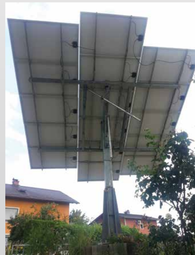
Solar tracker for 15 panels, with 16 panels, 3,75 kWp.
