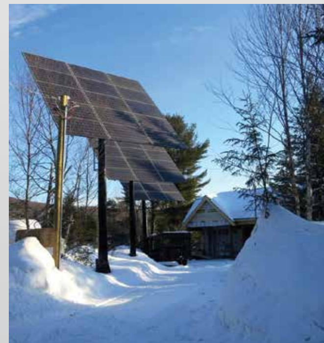
Solar tracker for 15 panels, 3,75 kWp.
