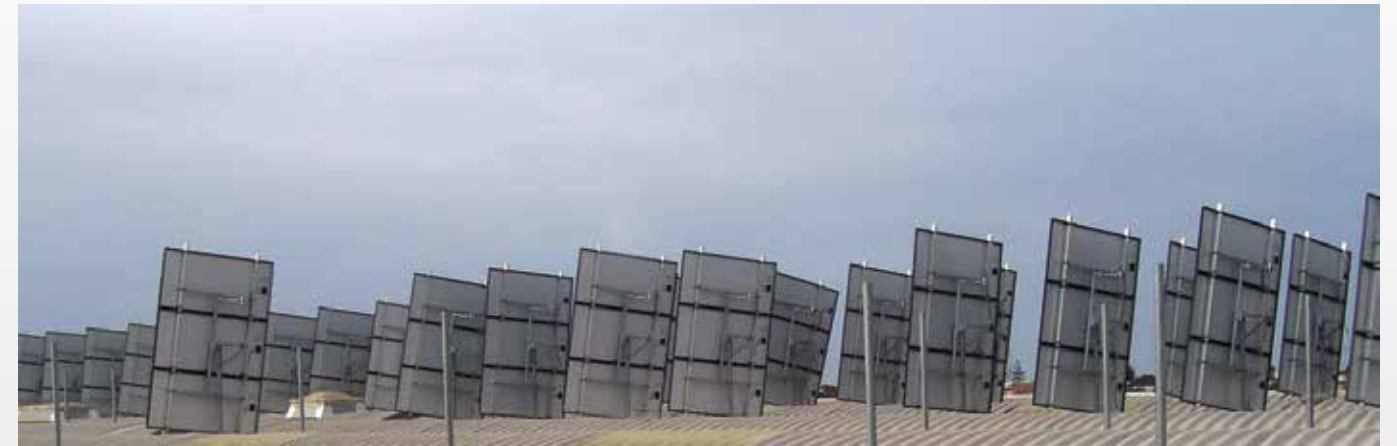
Power plant with an installed power of 58,50 kWp. Quantity of trackers: 78.
