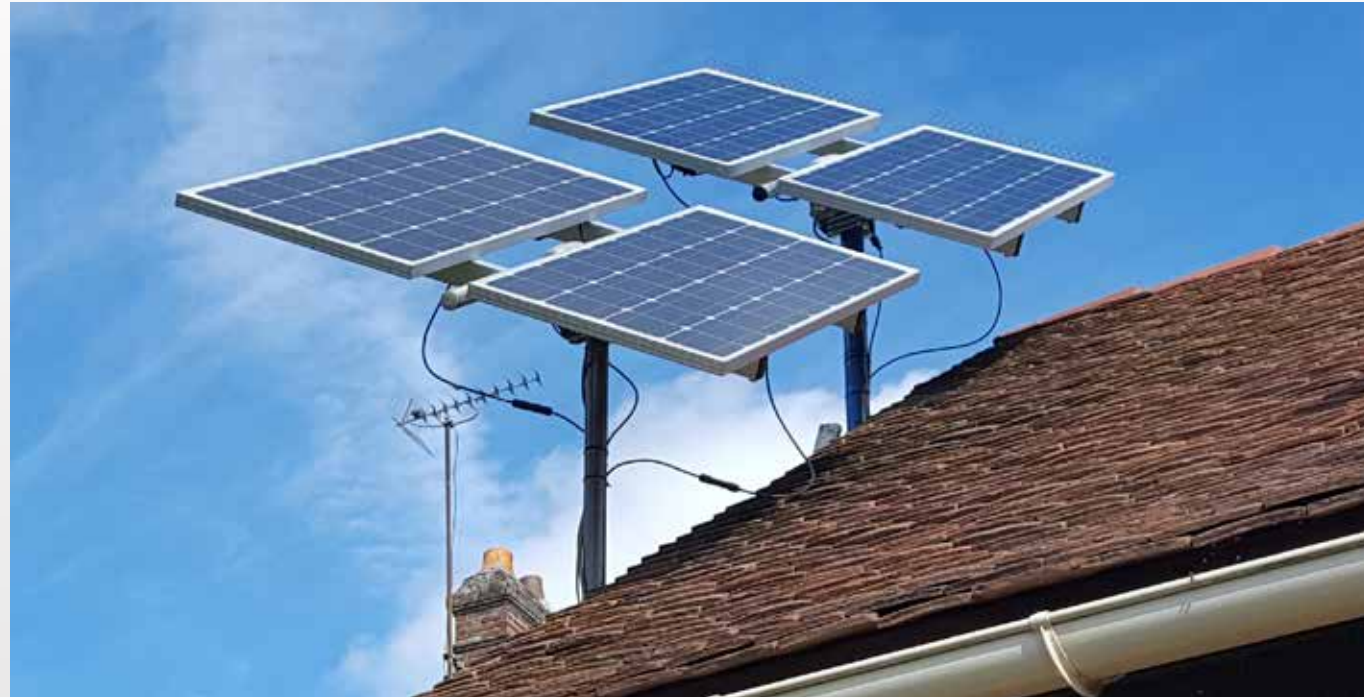
Solar tracker for 2 panel, 1,6 kWp. Quantity of trackers: 3.
