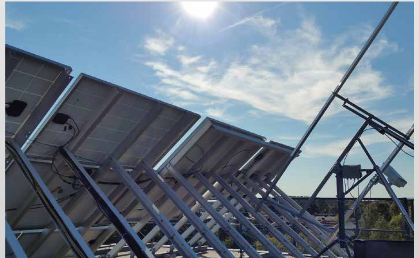
Solar tracker for 3 panels, 1,7 kWp. Quantity of trackers: 2.
