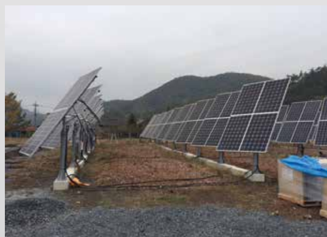
Power plant with an installed power of 58,08 kWp. Quantity of trackers: 44.
