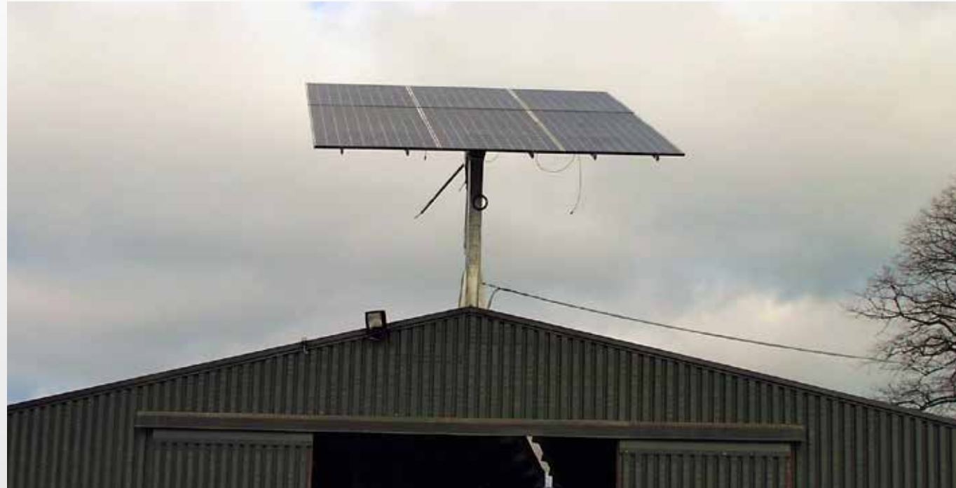
Solar tracker for 15 panels, 4,5 kWp.
