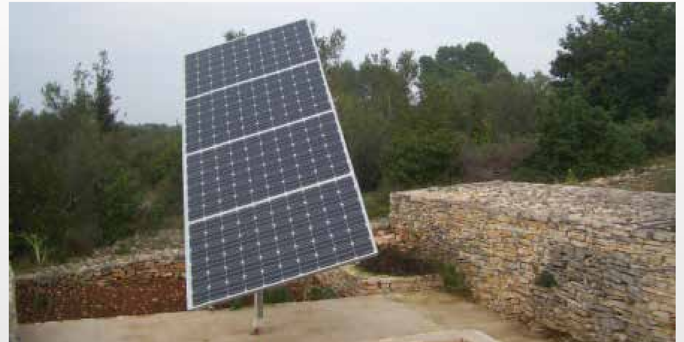
Solar tracker for 4 panels, 1 kWp.
