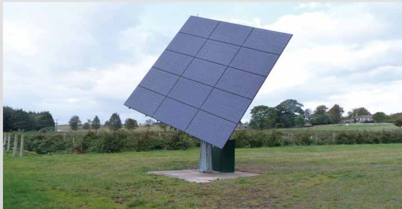
Solar tracker for 15 panels, 3,75 kWp.
