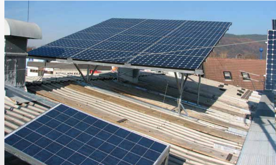
Solar tracker for 18 panels, 5 kWp.
