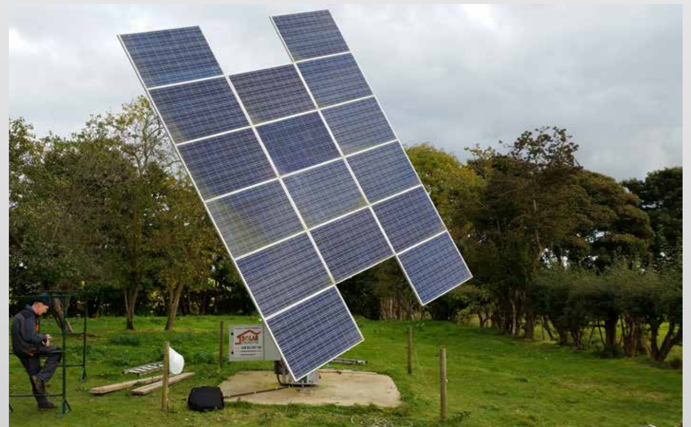
Solar tracker for 16 panels, 4,4 kWp.
