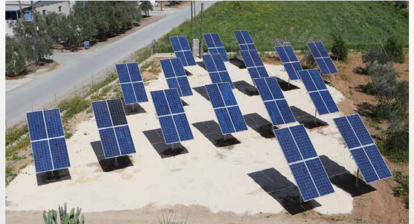
Power plant with an installed power of 20,00 kWp. Quantity of trackers: 20.
