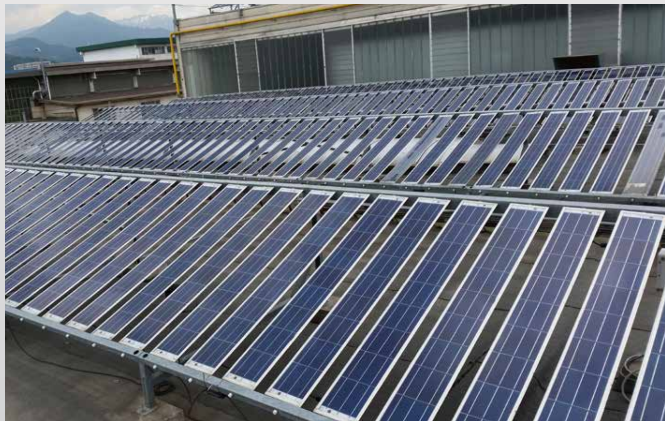
Power plant with an installed power 180 kWp. Quantity of trackers: 18.
