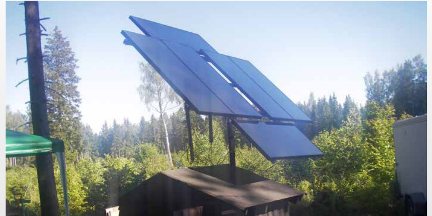
Solar tracker for 6 panels, 1,8 kWp.
