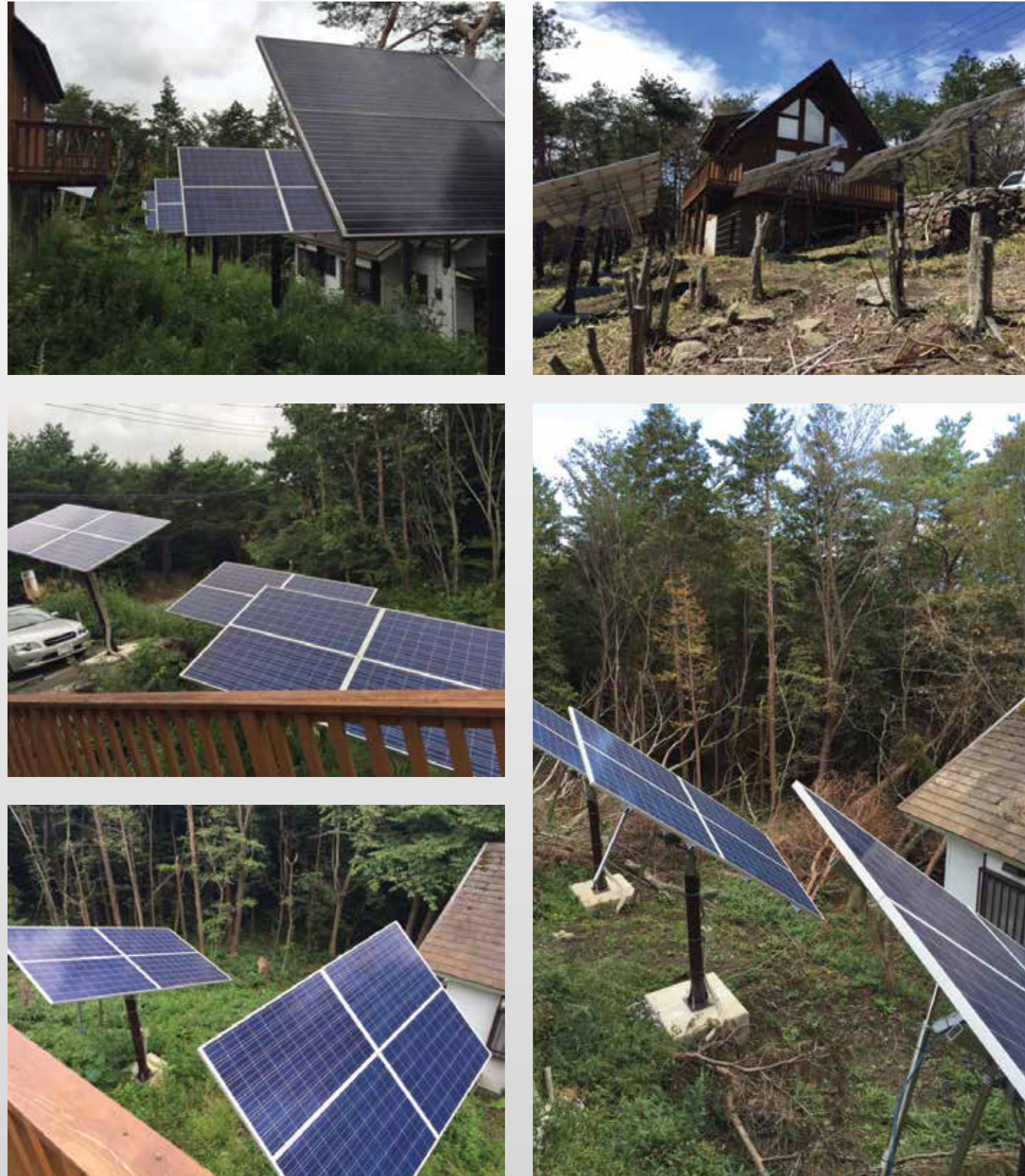
Power plant with an installed power of 10,56 kWp. Quantity of trackers: 8.
