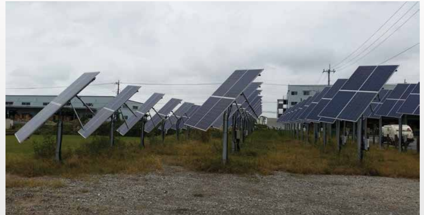
Power plant with an installed power of 66 kWp. Quantity of trackers: 50.
