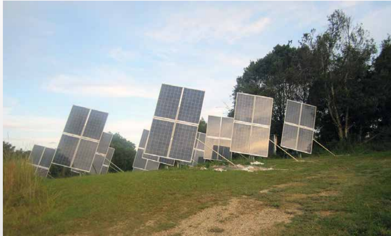
Power plant with an installed power of 12,00 kWp. 2.
