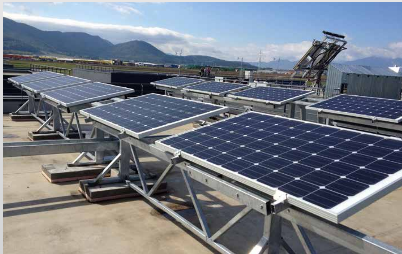
Solar tracker for 10 panels, 2,8 kWp. Quantity of trackers: 2.
