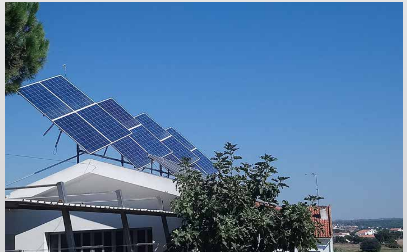
Solar tracker for 4 panels, 5,5 kWp. Quantity of trackers: 4.
