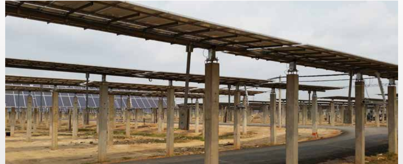
Power plant with an installed power of 120 MW DC.
