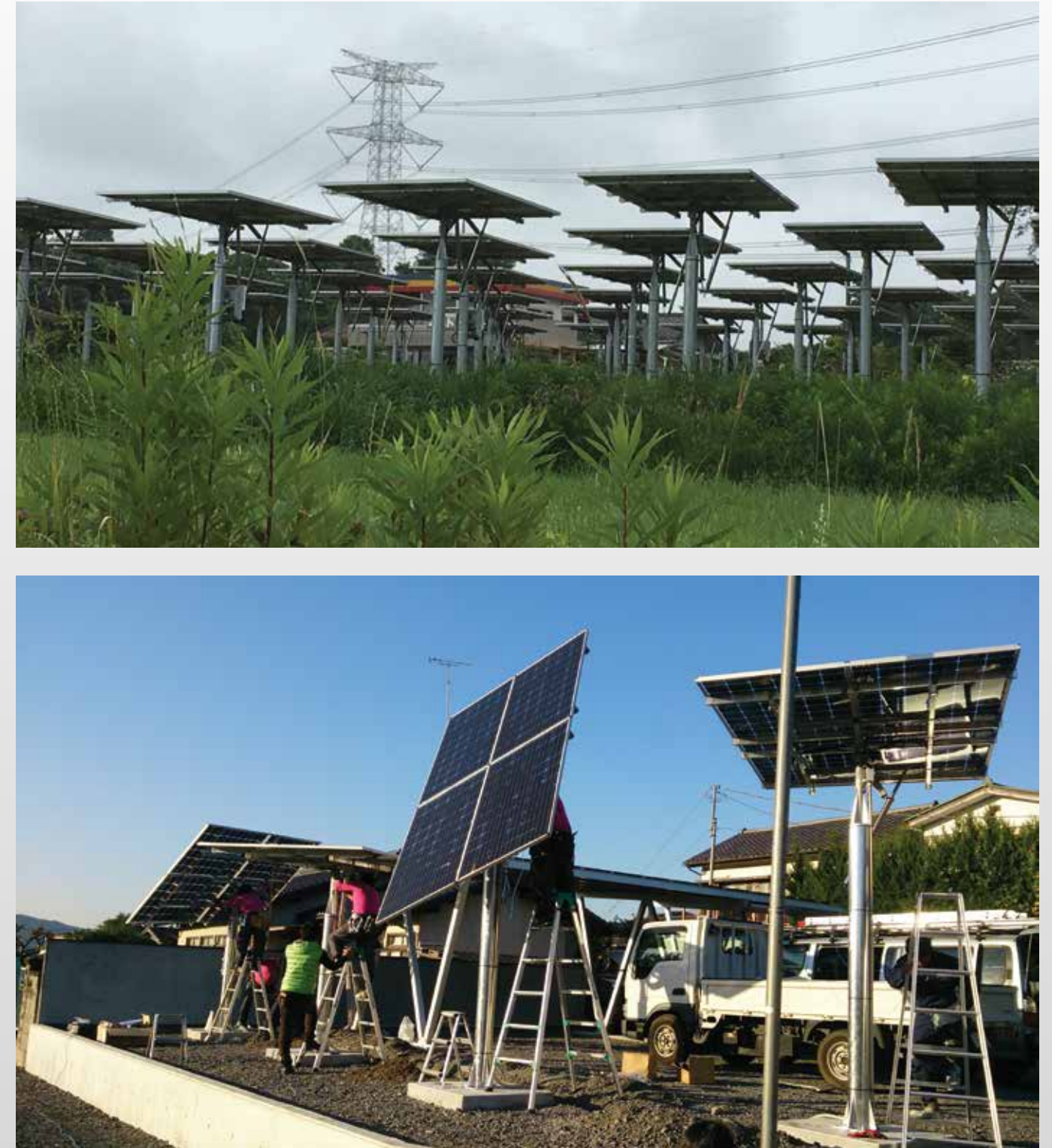
Power plant with an installed power of 66 kWp. Quantity of trackers: 50.
