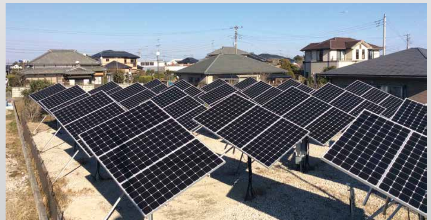
Power plant with an installed power of 58,08 kWp. Quantity of trackers: 44.
